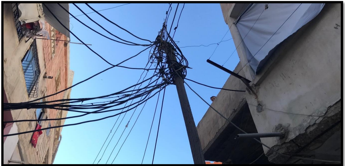
Figure 5.4 Difficulty in the installation and maintenance of the electricity in Corniche region
