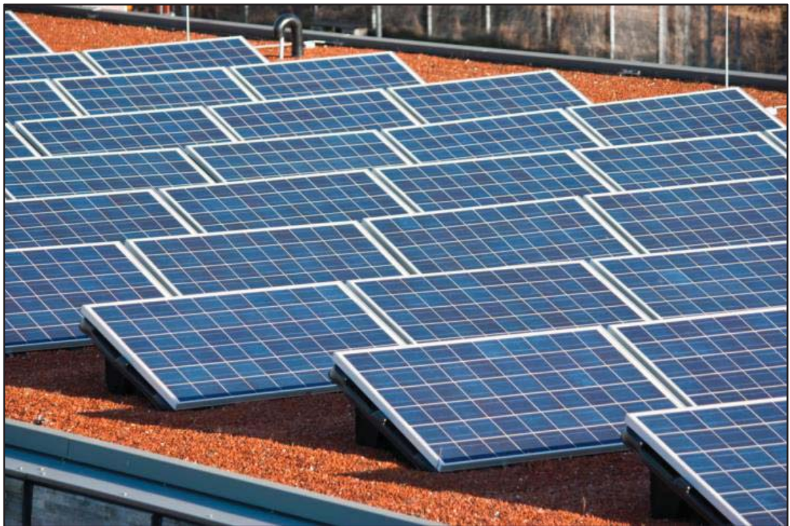
Figure 4.12: Photovoltaic panels installed on roof
